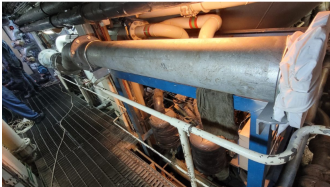
Return pipeline from ballast water treatment system back to existing ballast system onboard without obstructing main passageway.
