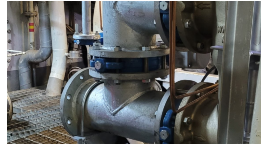
Ballast water treatment system 20 microns filter positioned with inlet and outlet pipeline installed.
