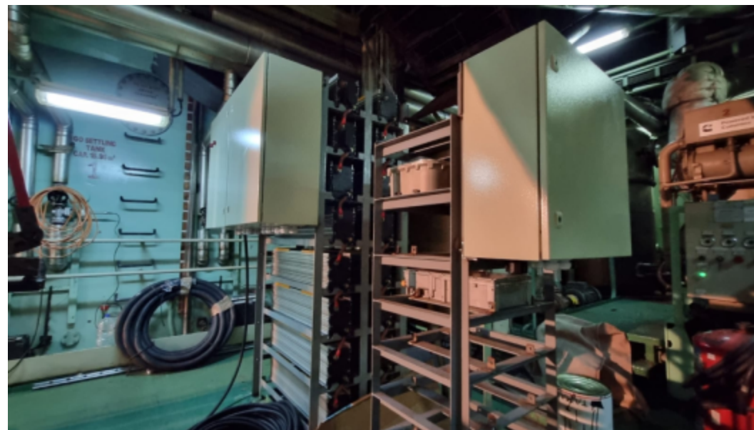
Electrical automation for an integration of a hybrid system onboard of a cargo vessel.
