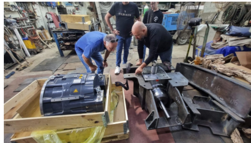
Electrical motor/generator installment for an integration of a hybrid system onboard of a cargo vessel.
